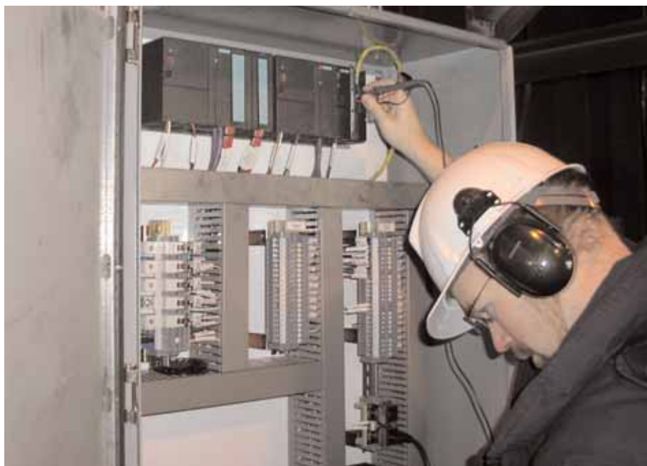
Thorough, correct start-up is the key to trouble-free network operation.
