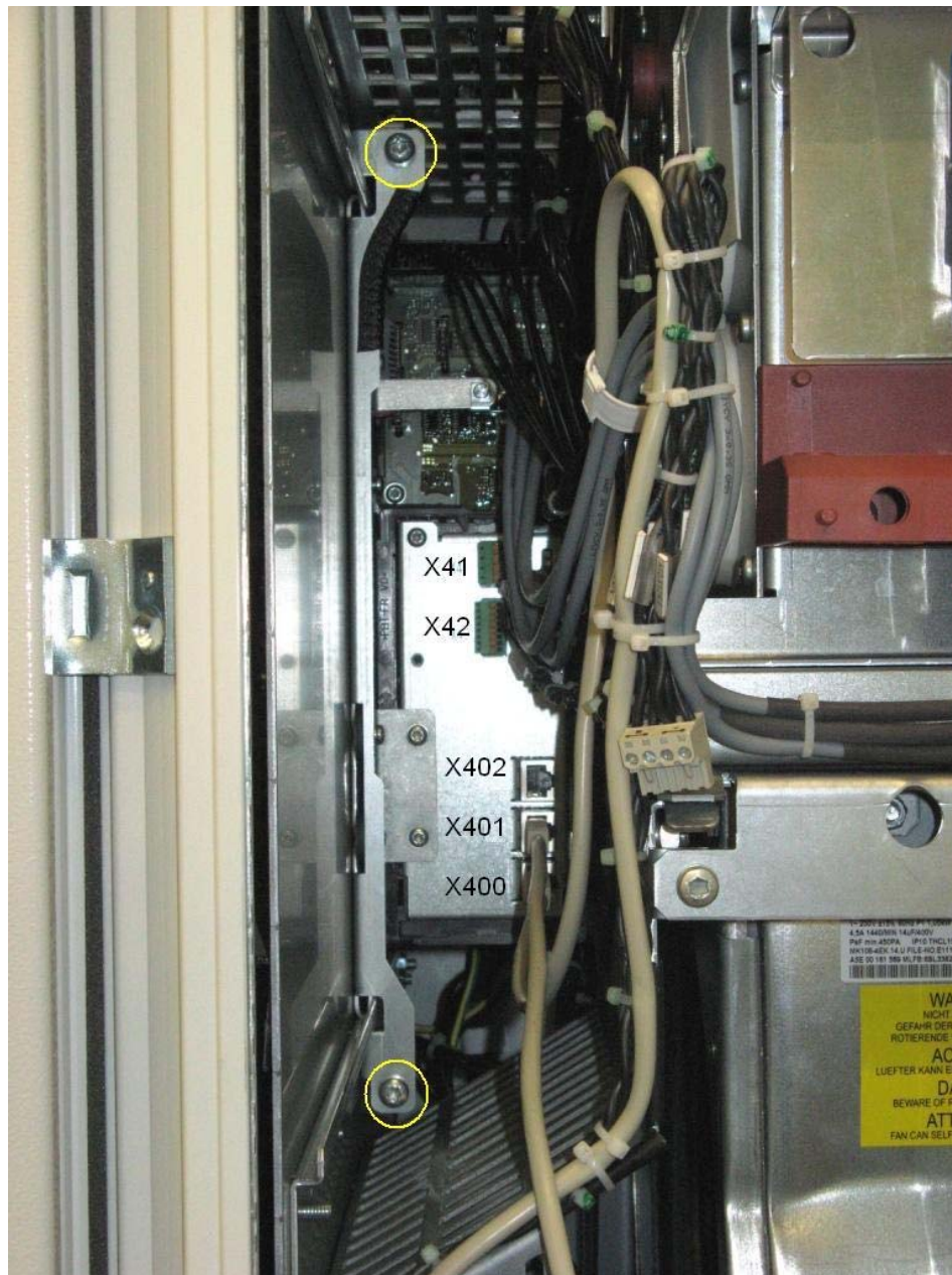
Fig. 3: Support plate with old control electronics module (CIB)
