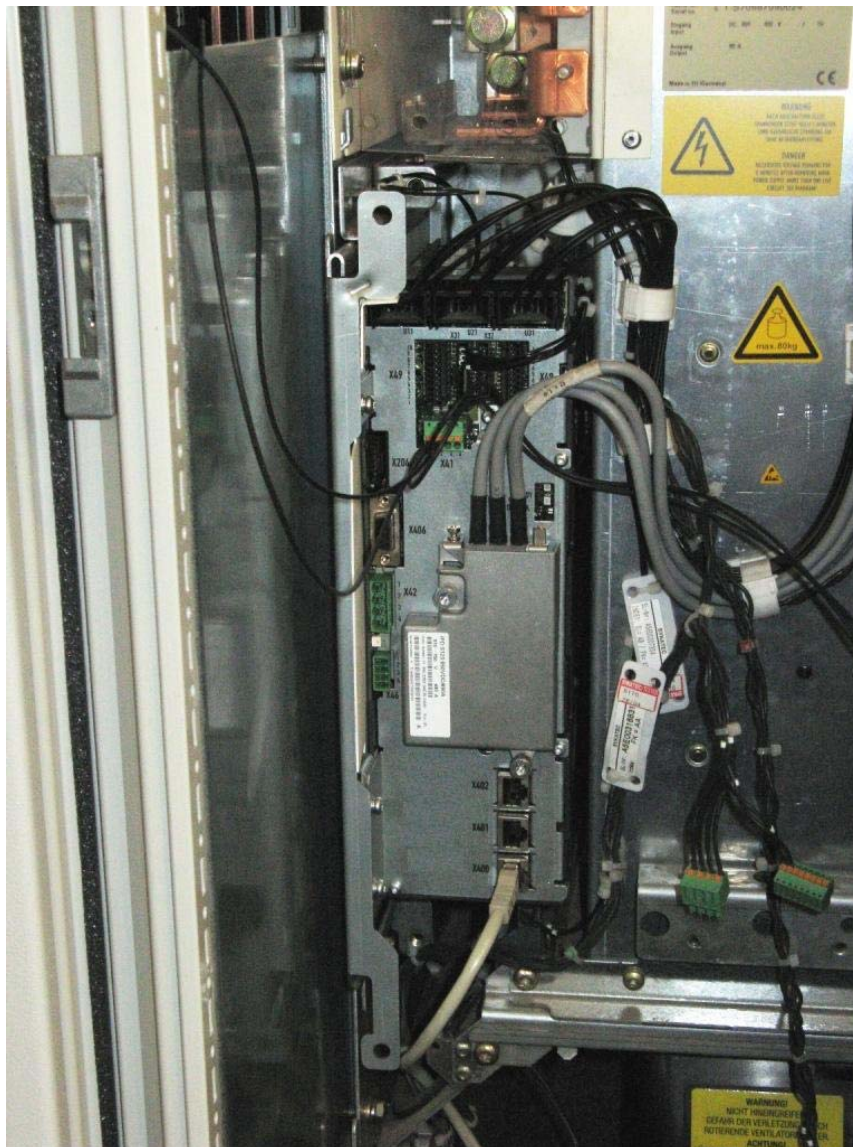
Fig. 5: New control electronics (CIM)
